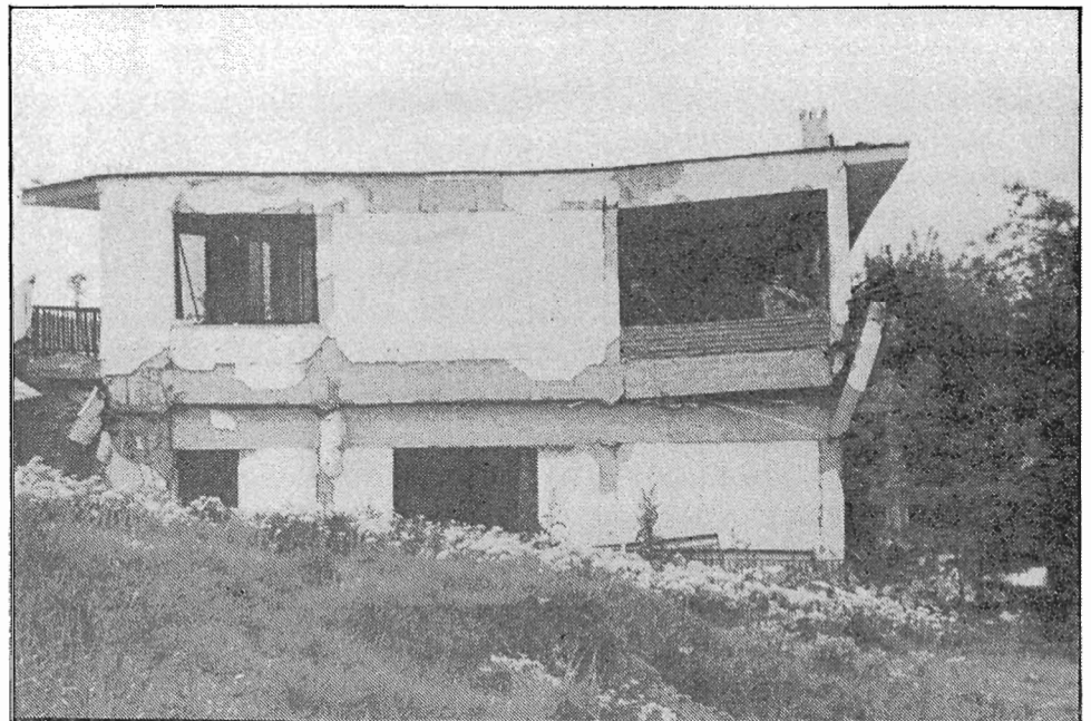
Plate 2: Collapsed middle floor of three-storey RC frame building outside Grevena.
