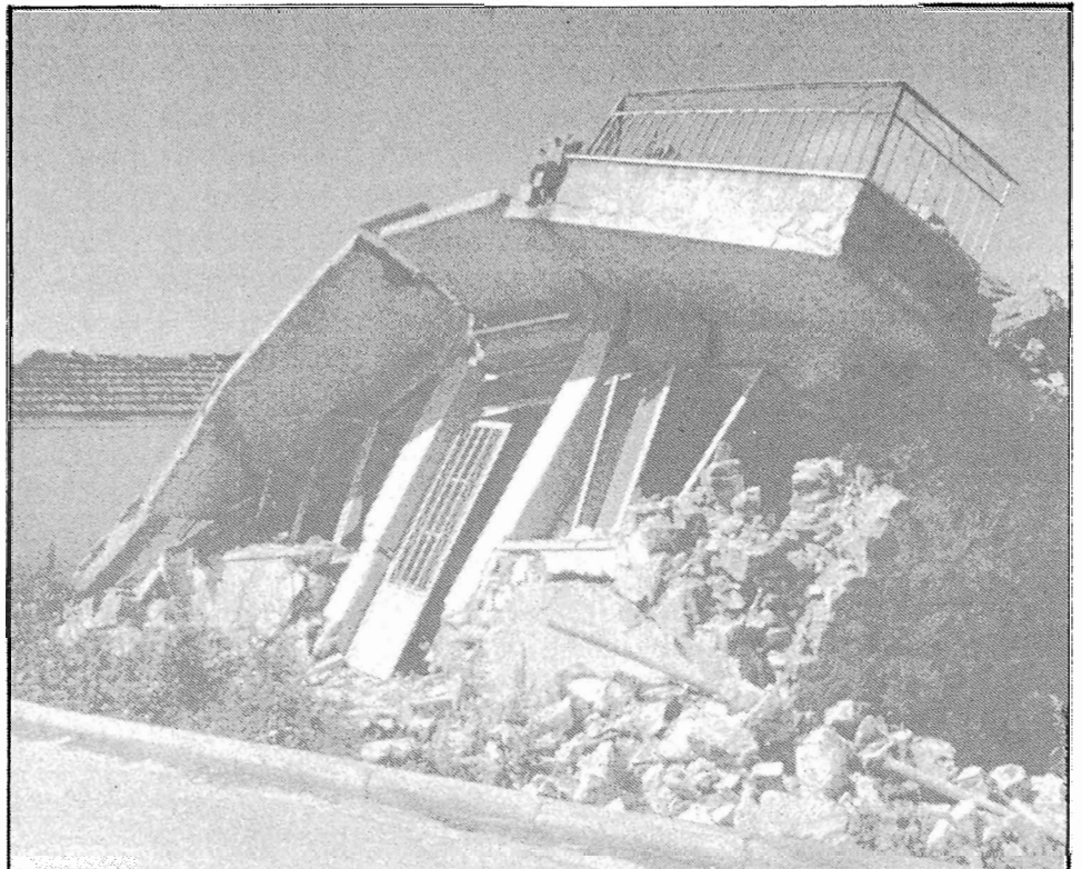
Plate 1: Collapsed two-storey house in Kalamitsi.
